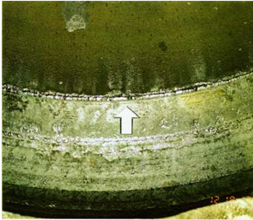
Photo 2: Minor leakages, and “fans”
