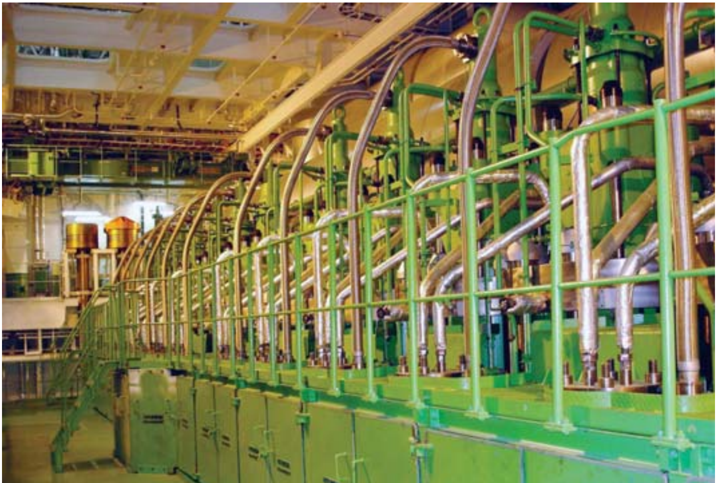
Fig. 1: General view, 12K98ME installed in a container ship
