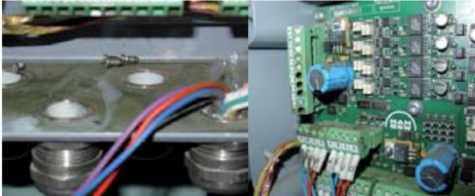
Fig. 36: PCB, metallic dust from untightened (unused) screws
