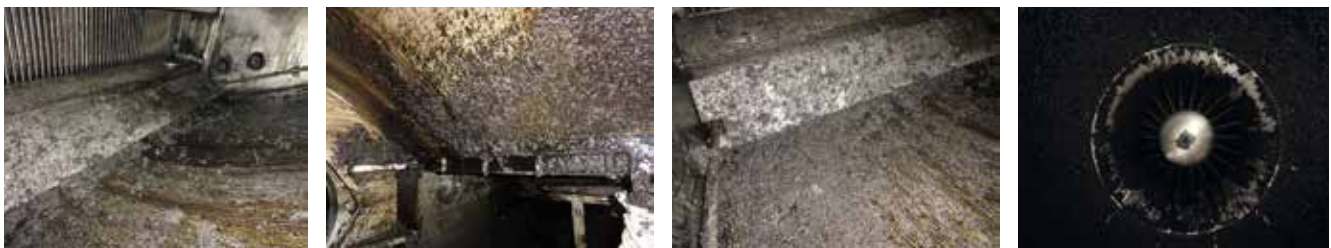
Fig. 41: EGR-blower suction chamber greasy oily sooth lumps accumulated
