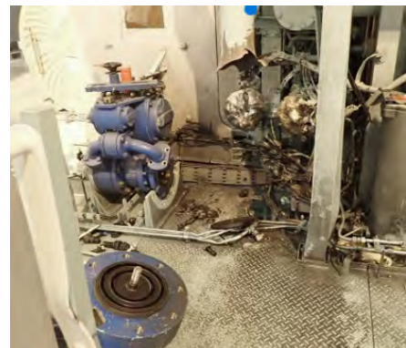
Ruptured starting air manifold
