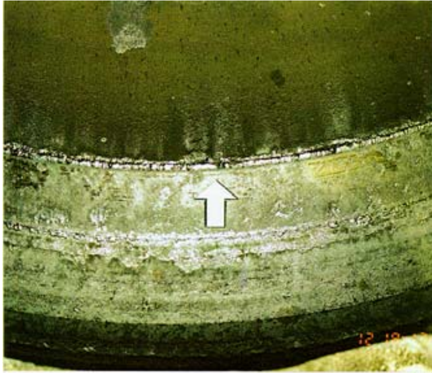
Photo 2: Minor leakages, and “fans”
