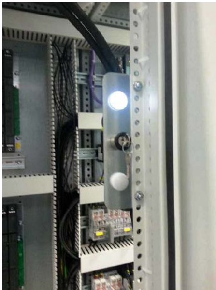
Figure 6-13: Key switch for PLC switch over
