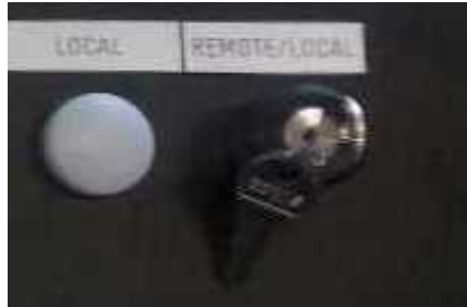
Figure 6-4: Controls for local / remote on CCD
